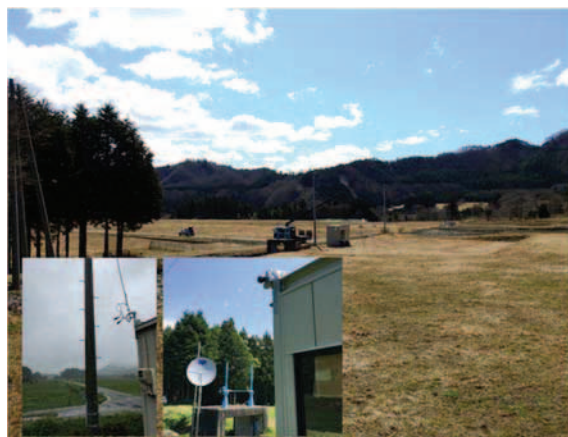
Fig. 2. Construction of transmitter station at project site in exclusion zone. (© Hill Hiroki Kobayashi)
