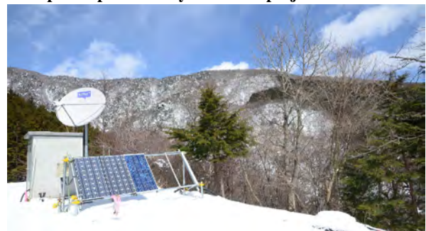
Figure 8. Data Communication System: Satellite Internet dish, solar panels, and control house in Cyber Forest project site.
